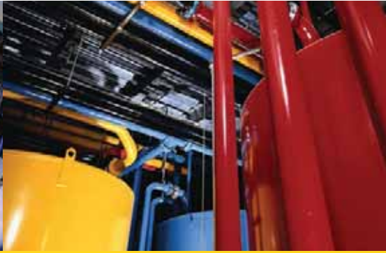
Compressor Rooms and Main Ring Applications
